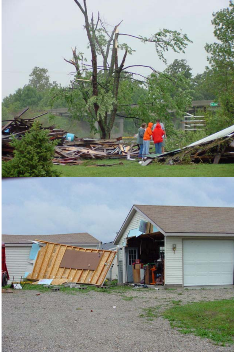
Tornado damage, Northwestern Delaware County, September 20, 2002. Photos by the applicant
